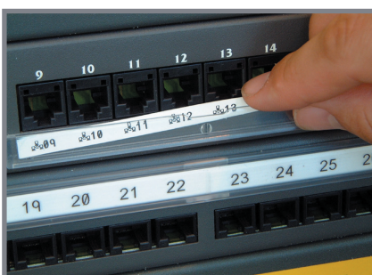
Punch Block & Patch Panel Labels
